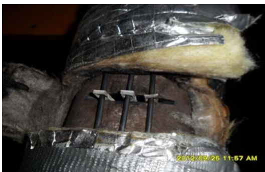
Fig.1. The placing of the samples in the exhaust pipe of the AV00 boiler
