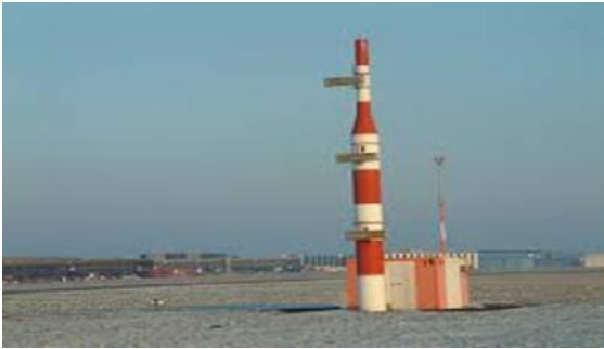
Fig 1.1 Glide Path beacon of the ILS system
